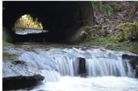
What was once a concrete apron designed to help salmon navigate this culvert has since eroded into a sharp, jagged concrete lip that creates a hazard for fish as they try to move upstream.
